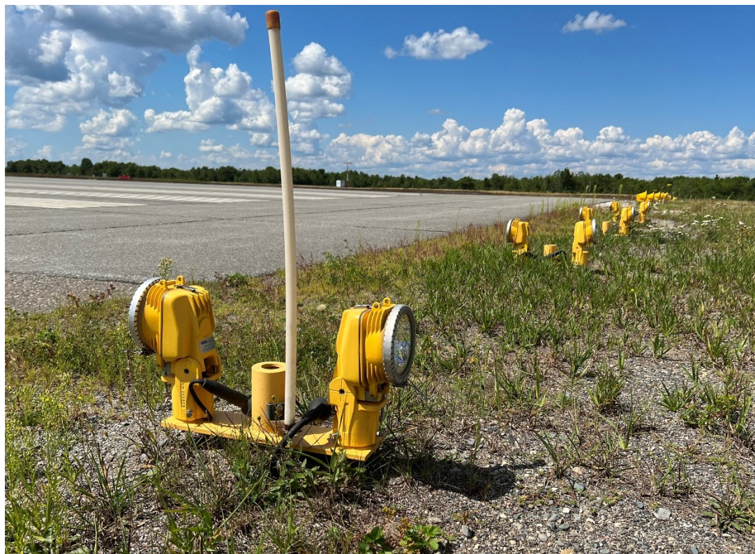
Figure 26 - Runway End and Threshold Lights on Runway 22
