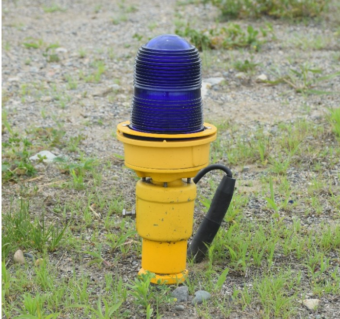
Figure 30 - Taxiway Edge Light
