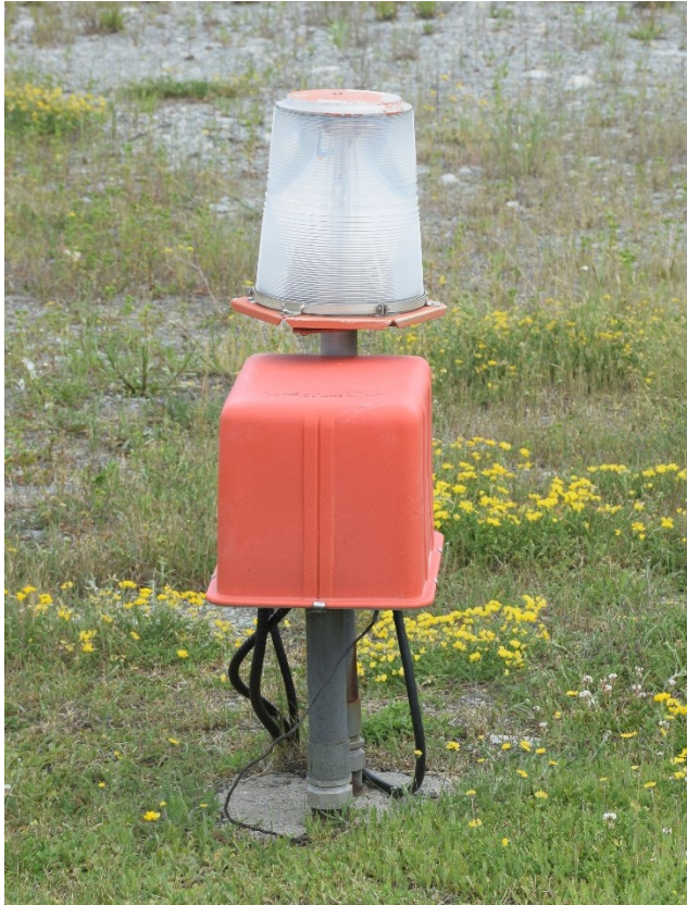
Figure 40 - Omni-Directional Approach Light (ODAL) Unit
