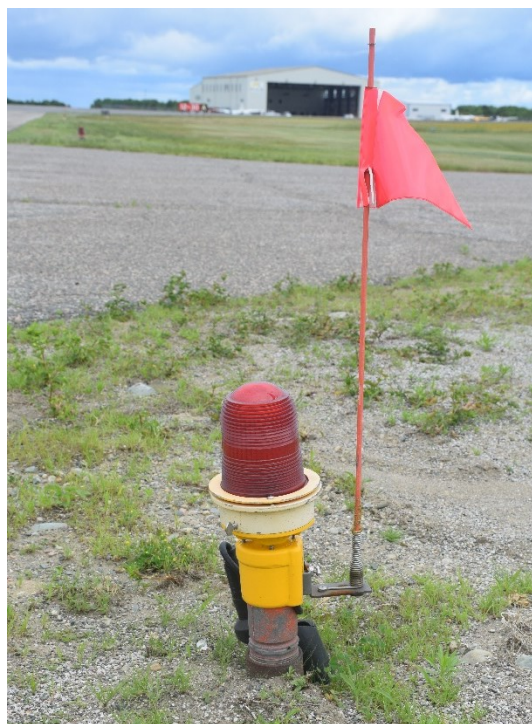
Figure 32 - Service Road Light
