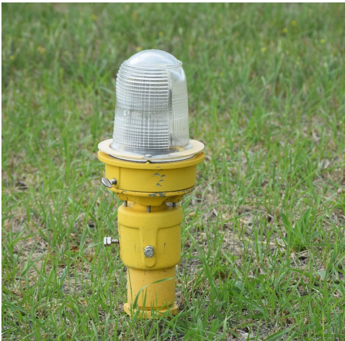
Figure 22 - Runway Edge Light
