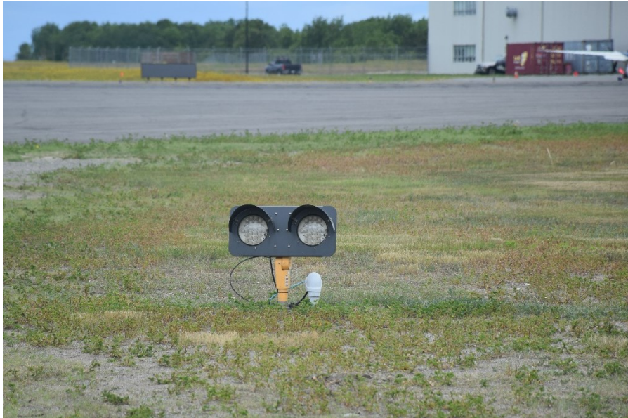
Figure 14 - Runway Guard Light
